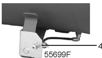
Condensate drain valve on air receiver
