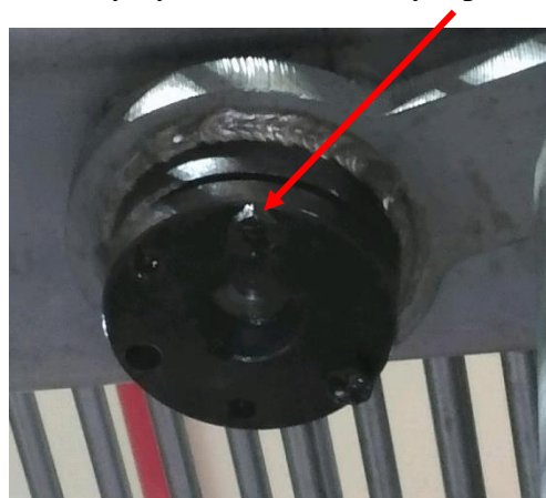
Sign of leaky hydraulic motor oily taper lock
