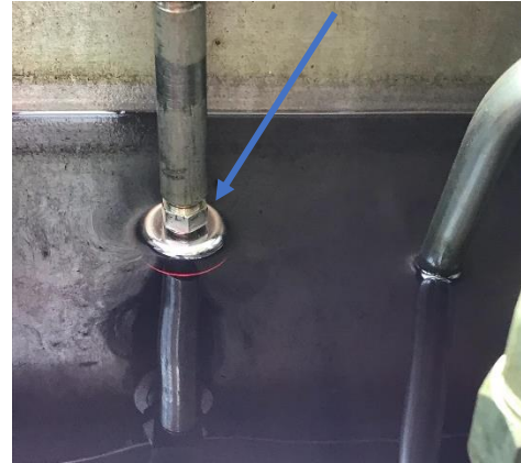
Example of correct hydraulic level
