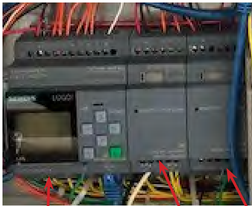
PLC Digital Extension Analog Extension
